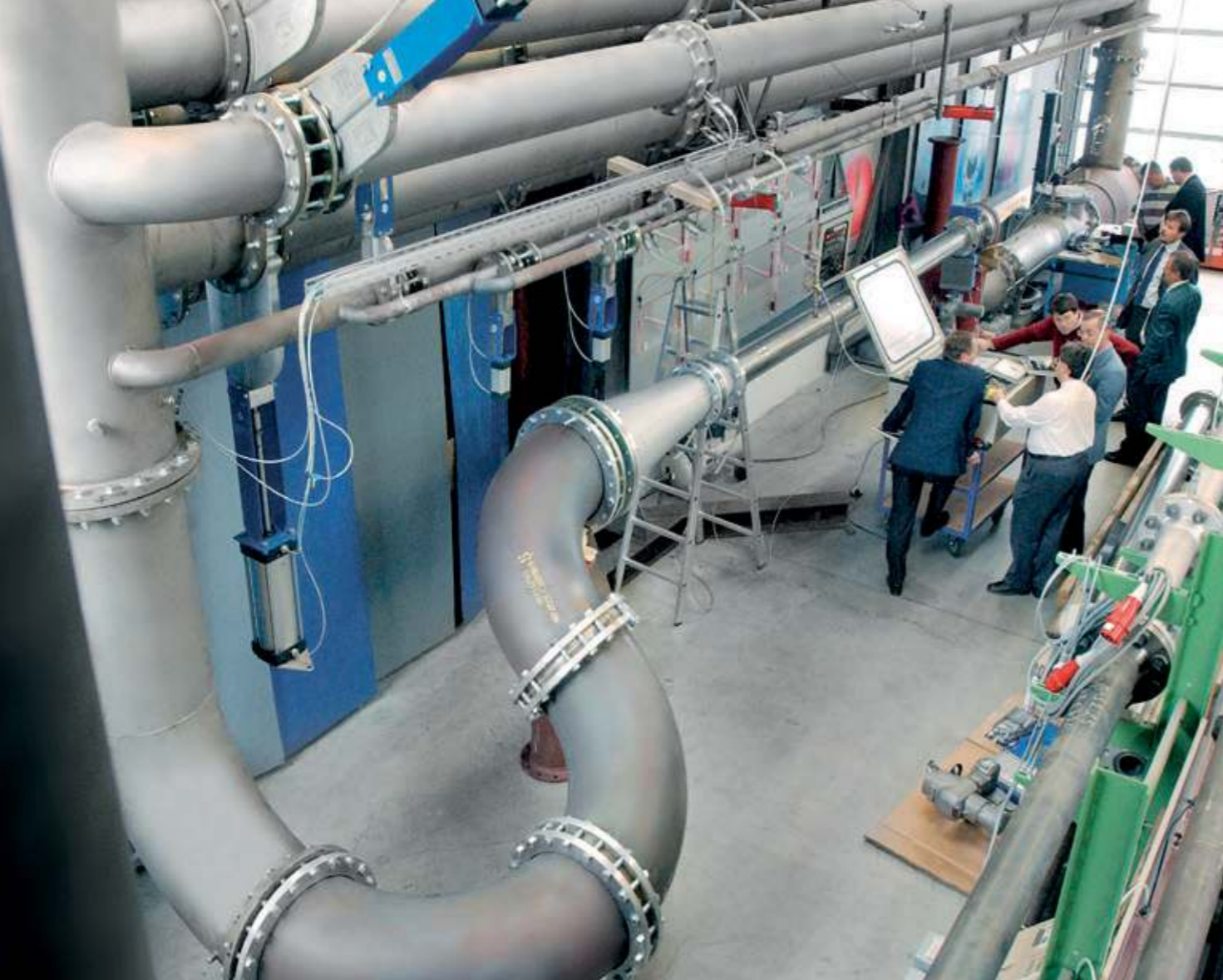
Factory approval testing (FAT) of the VACOMASS® air supply systems for the municipal sewage treatment plant of Vienna in our CAMASS® calibration centre. Due to the precise simulation of the field operating conditions and its piping layout during the calibration of the VACOMASS® systems, an accuracy of 1.5% of the airflow reading could be guaranteed despite the difficult piping.
